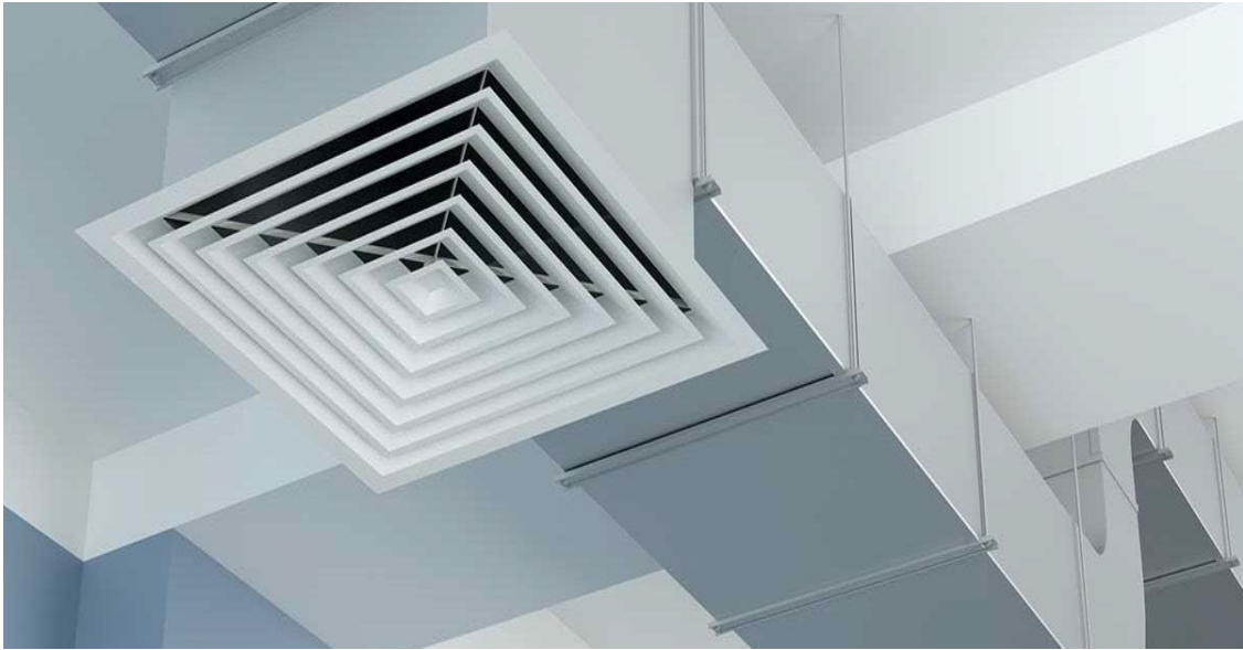
Fig. 3.1.14: HVAC vents and ducts
