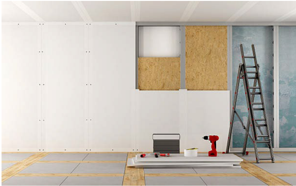
Fig. 6.2.7: Ensuring the installation of supporting structures for correct alignment of the panels
