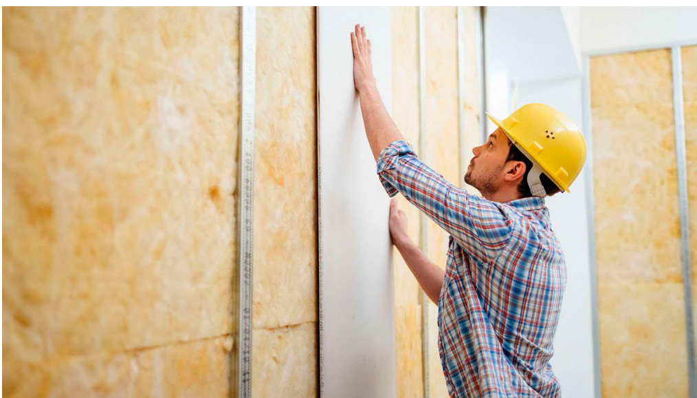
Fig. 6.2.9: Checks for the alignment of panels and joints ensuring verticality of the end wall
