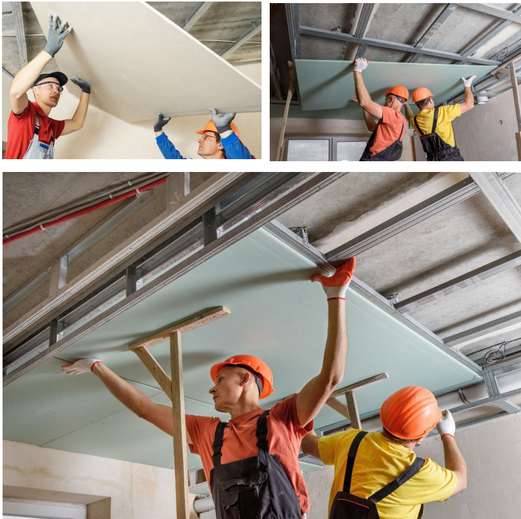
Fig. 3.2.21: Installation of framework and gypsum boards at the correct height and alignment
