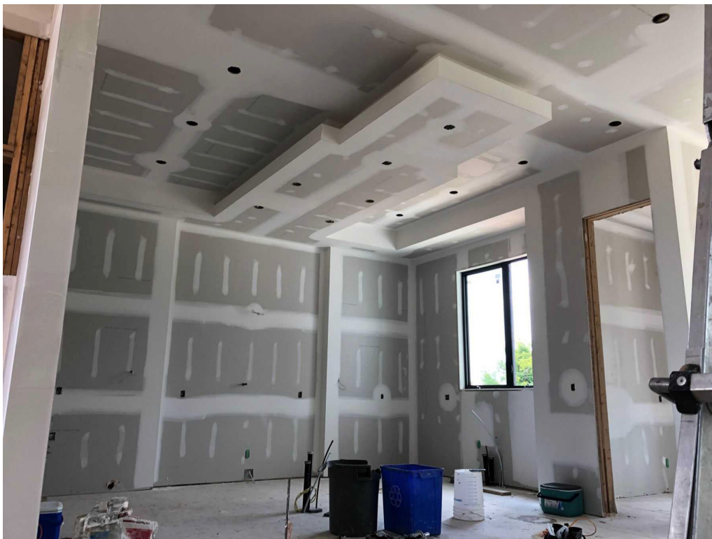
Fig. 6.2.5: Proper spacing between the bottom end of the panel and the floor
