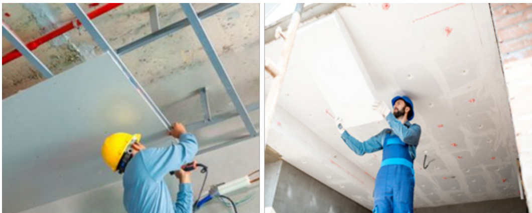
Fig. 3.1.38: False ceiling installations
