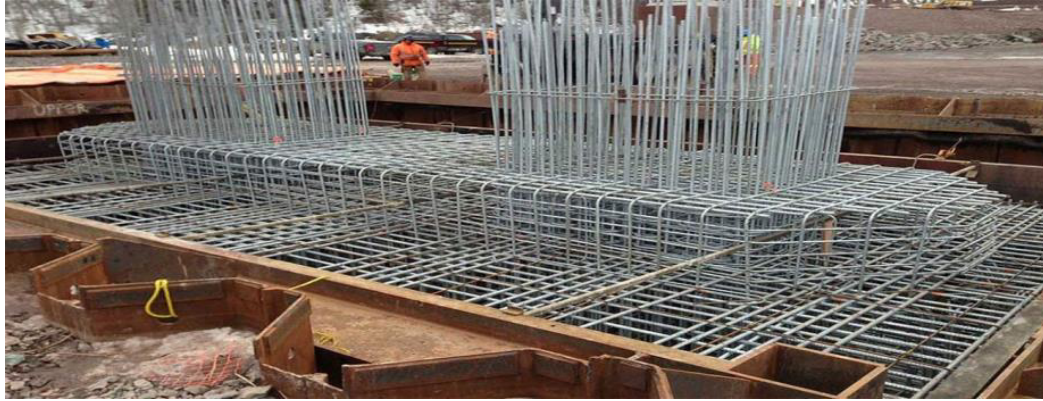
Fig. 6.3.4 Initial fixing ties to fabricate the required cage for reinforced concrete structures
