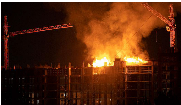
Fig. 9.2.3 Fire at Construction Site
