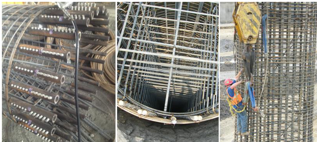
Fig. 6.3.4 Initial fixing ties to fabricate the required cage for reinforced concrete structures
