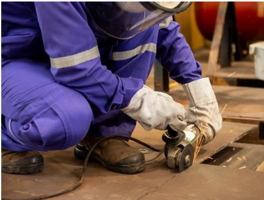
Fig. 4.2.26: Wear non-conductive safety gear
